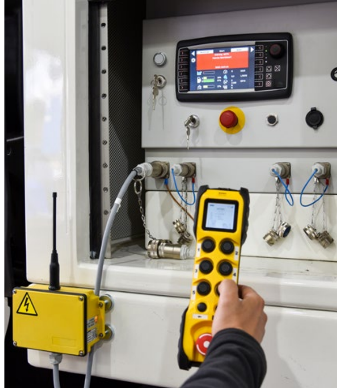
Connected transceiver at the control cabinet
