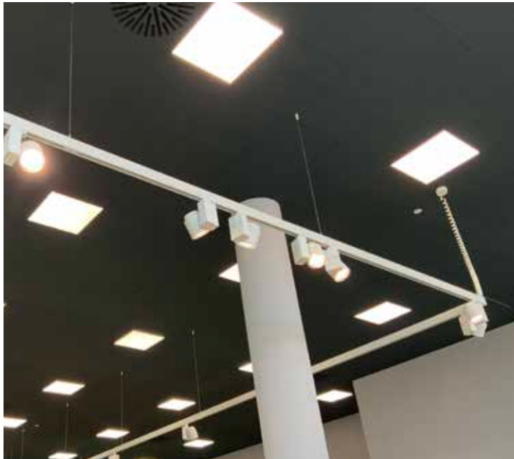
Lighting with rail system
