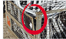
The hinged front wall panel can no longer be opened or closed.
